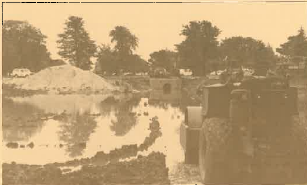
Construction of the detention ponds is already in progress on the Glenview Naval Air Station Base. The project is a fine example of the cooperation between the Village and the Navy Base.
