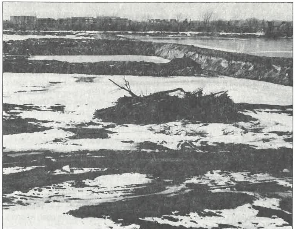
This is a photograph of the reservoir under construction in Deerfield, on the southwest corner of Lake Cook and Pfingsten Roads. The reservoir system improvements will help reduce the possibility of overbank flooding in Glenview.
