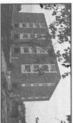
FALL, 1987: Top soil has been spread, and curbs for driveway are ready to be poured. (Landscaping was completed before snowfall.)
