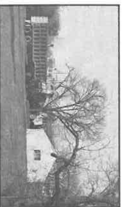
Demolition contractor takes down the landmark farmhouse, and is about to begin razing an outbuilding. (Note old oak tree in left foreground — it will be saved.)
