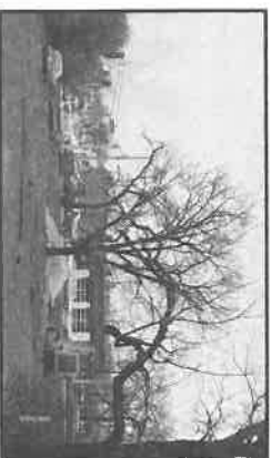
Buildings razed and debris carried away, tractor levels site and prepares to cover low spots with gravel. All views are from the south (Dewes Street) side.
