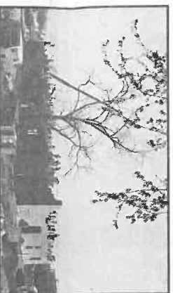
WINTER, 1987: Patten House begins taking shape, brick by brick, in classic from-the-ground-up masonry method.
